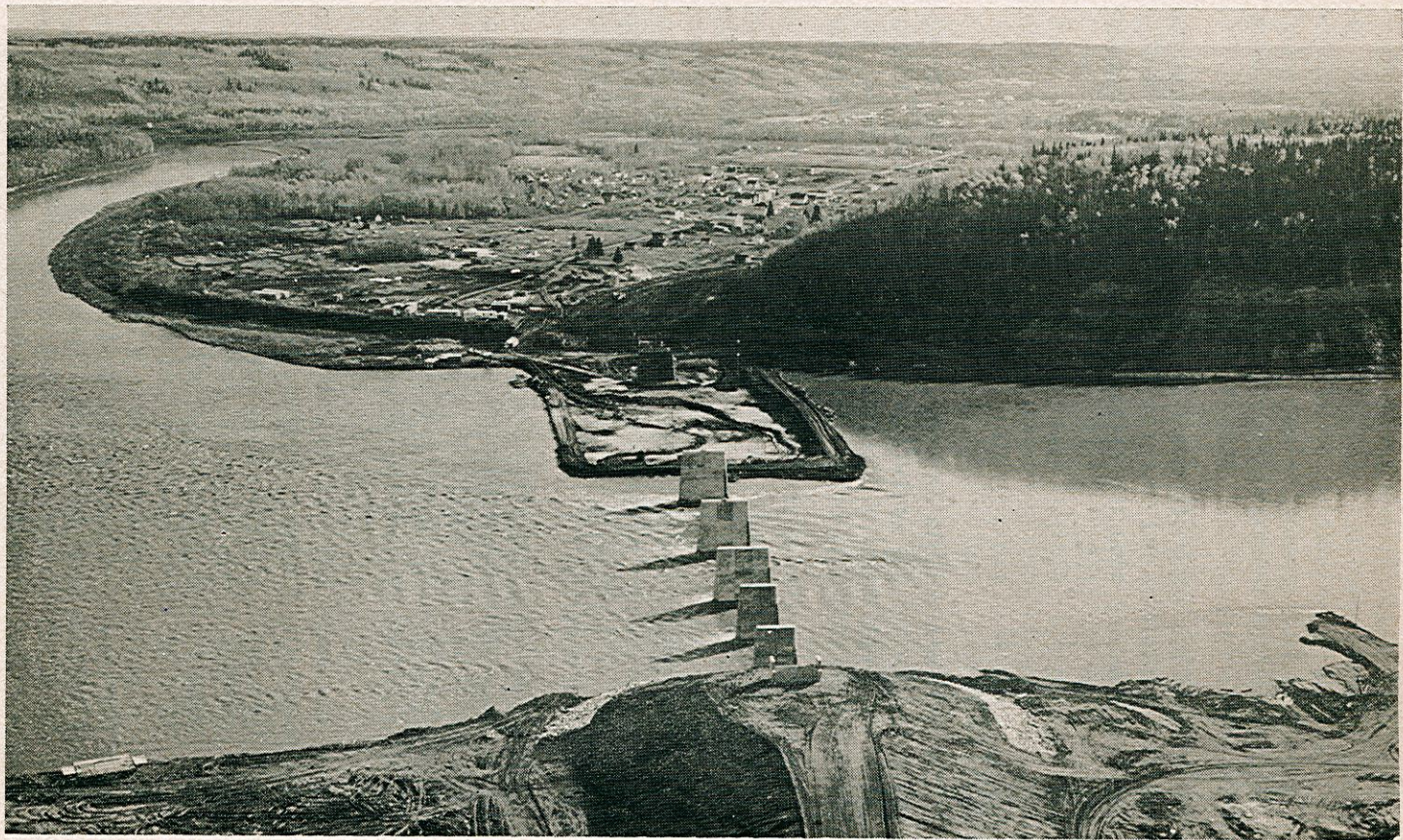
Bridge construction across the Athabasca River at Fort McMurray to serve the Great Canadian tar sand development
